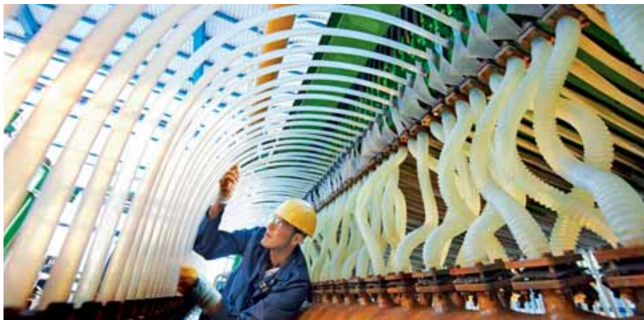
Plant assistant Jörg Bähler checks the oxygen inlet pipe of the plant at Bayer’s Brunsbüttel site that uses the oxygen depolarized cathode technology.
